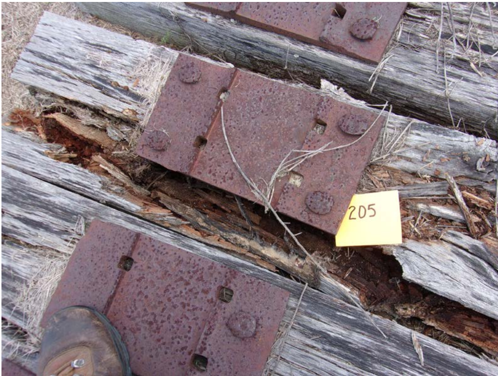
Figure 11 - Tie #205 with extensive decay.
