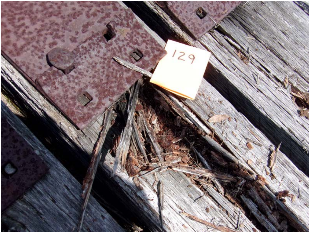
Figure 9 - Tie #129 with heavy decay.
