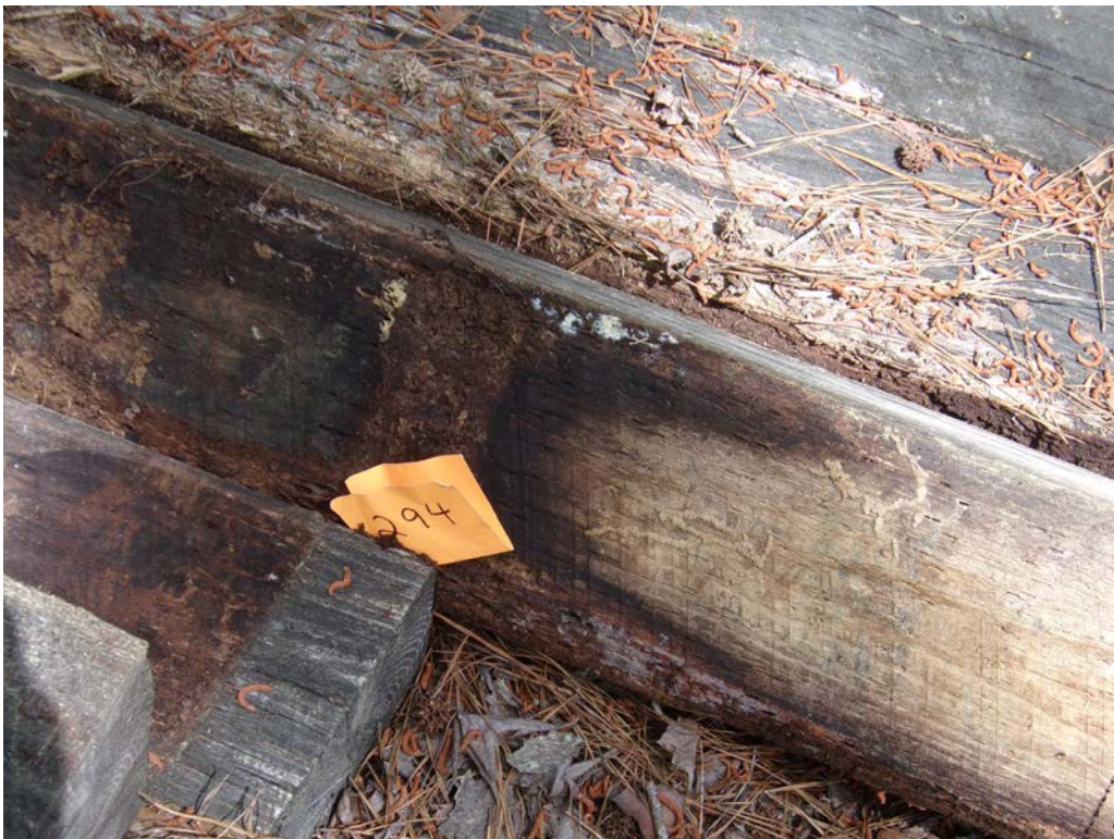
Figure 5 - Tie #294 with light decay and trace termite attack.
