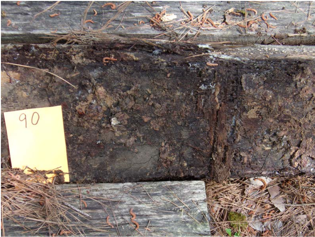
Figure 4 - Tie #90 with light decay and termite damage.
