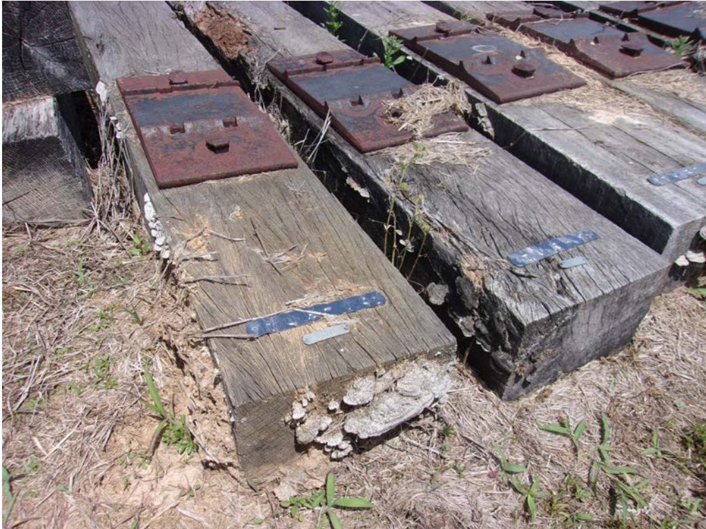
Figure 6 - Ties #4-#6 with decay and fringing bodies.
