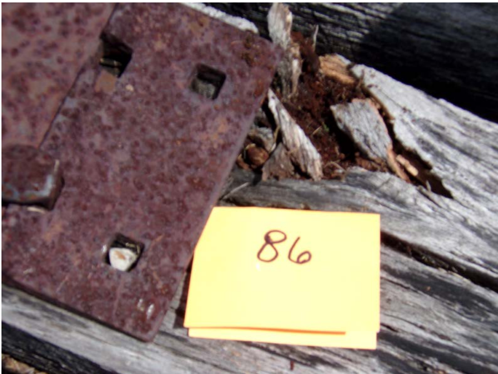
Figure 7 - Tie #86 with decay.
