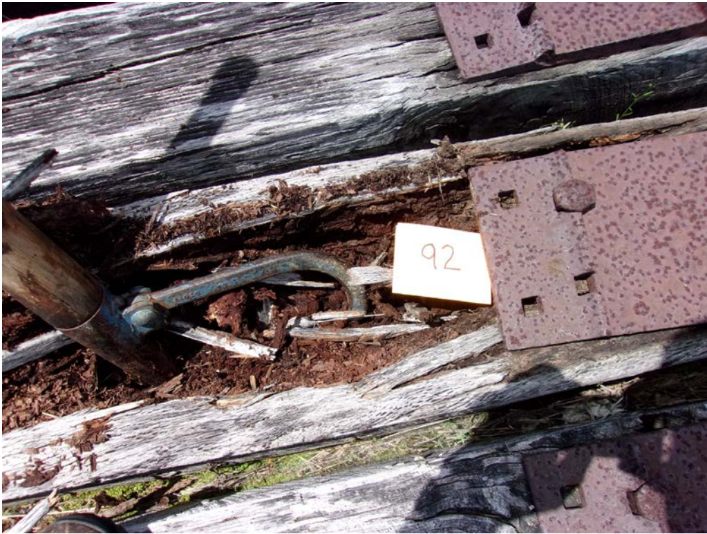
Figure 8 – Tie #92 with extensive decay.
