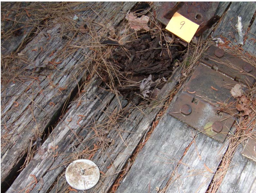
Figure 3 - Tie #9 showing extensive decay.
