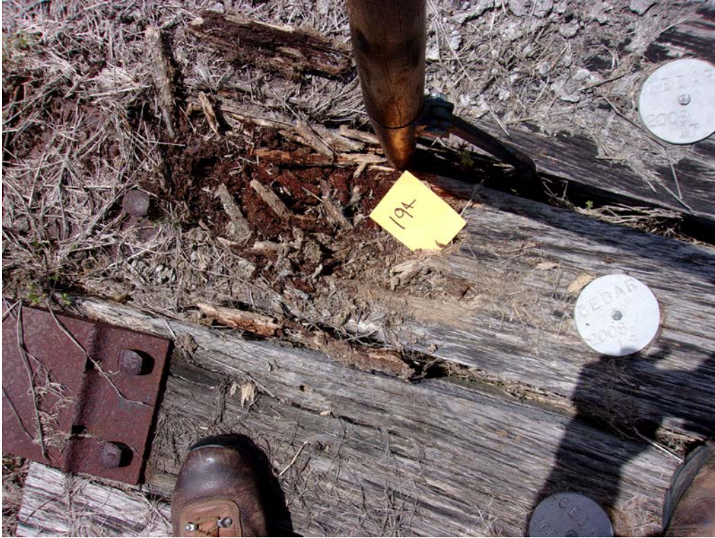
Figure 10 – Tie #194 with heavy decay.
